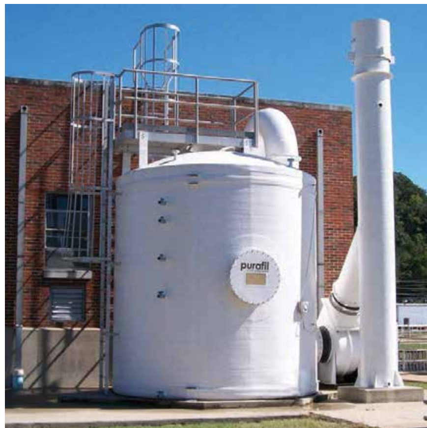
Moccasin Bend Wastewater Treatment Plant, Chattanooga, Tennessee
