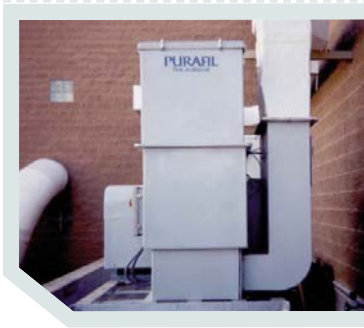
PURAFIL ESD TUB SCRUBBER SYSTEM
