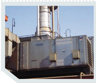
PURAFIL DEEP BED SCRUBBER AT TUPRAS IZMIT REFINERY IN TURKEY
