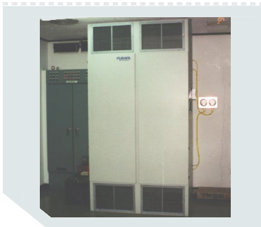
PURAFIL CORROSIVE AIR SYSTEM
