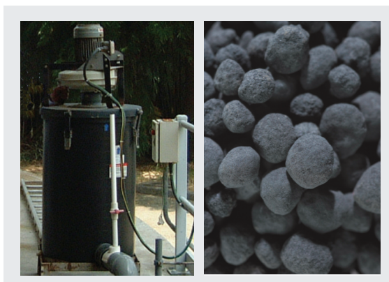
PURAFIL™ DRUM SCRUBBER 100 INSTALLED AT THE WANCHAI WEST PRELIMINARY SCREENING PLANT
