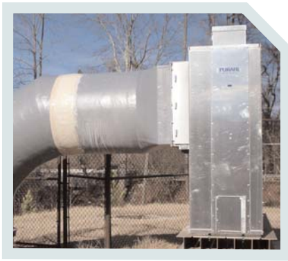
PERMANENT PURAFIL® ESD DEEP BED SCRUBBER AT THE JOHNSON FERRY ROAD #2 LOCATION
