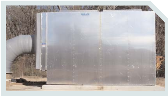
PERMANENT PARALLEL BED SCRUBBER AT THE ROSWELL ROAD #2 LOCATION
