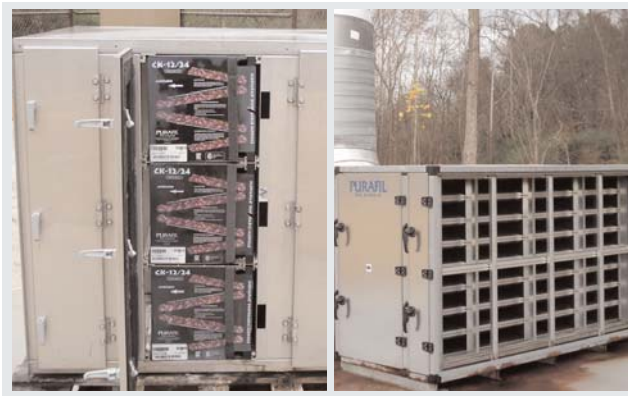
TEMPORARY PURAFIL® SIDE ACCESS SYSTEM WITH CK-12 MODULES AT THE JOHNSON FERRY ROAD #2 LOCATION
