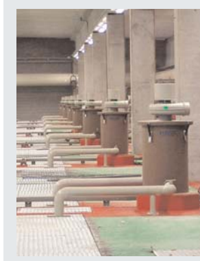
SEVERAL PURAFIL® ESD DRUM-SCRUBBER INSIDE THE BESOS WWTP WORK TOGETHER TO REMOVE THE ODORS FROM THE CITIES' WASTEWATER.
