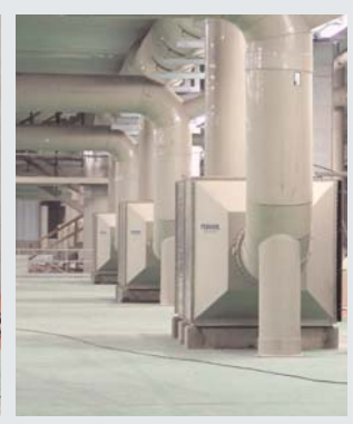
PURAFIL® SIDE ACCESS SYSTEMS WITHIN THE BESOS WWTP
