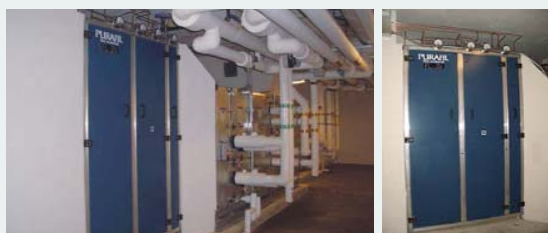
A TEAM OF PURAFIL AND TRANE ENGINEERS WORKED CLOSELY TO INCORPORATE SIX PSA'S INTO TRANE AIR HANDLING UNITS INSTALLED IN MECHANICAL ROOMS AT THE ARCHIVES.
